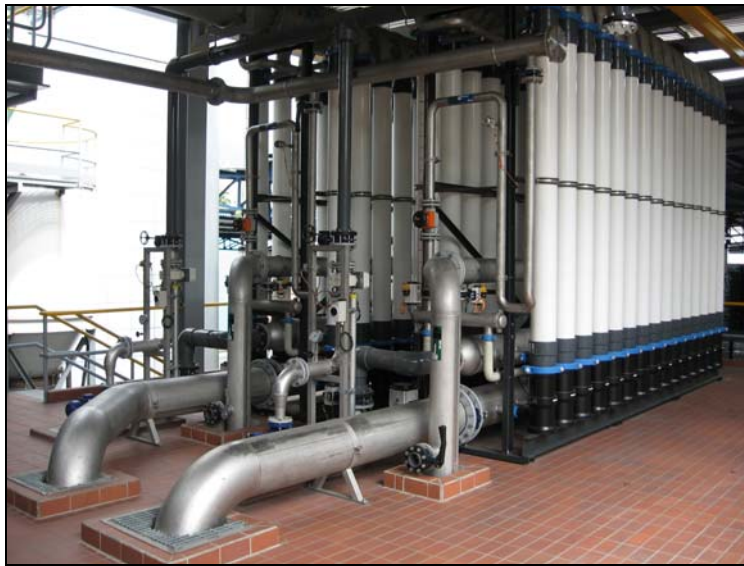
Fig.1 – Ultra-filtration System in Operation
