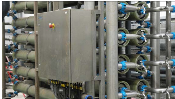
Fig.1 – Reverse Osmosis System in Operation
